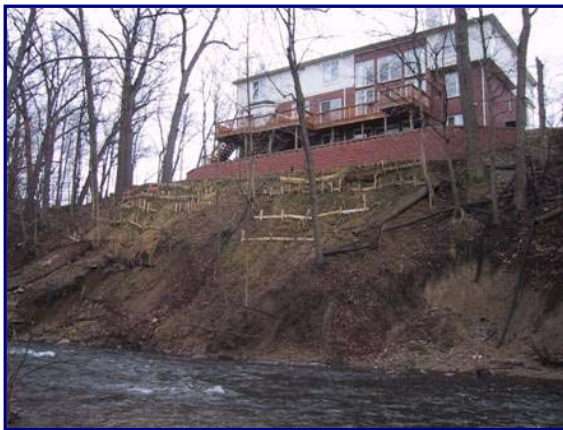
Figure B.3. Erosion due to channel migration is threatening this property in the City of Rochester Hills (photo taken in 2002).
