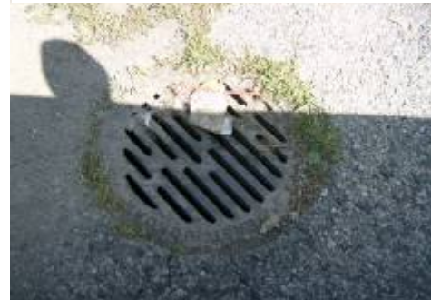
Figure 21: Garbage on Drain
