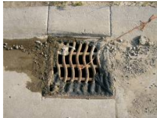
Figure 20: Sediment going to Drain
