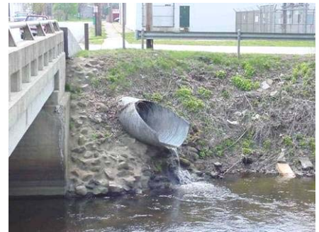
Storm Sewer Outfall w/ Dry Weather Flow – possible illicit discharge
