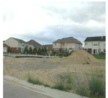
New Development in a Suburban Area of the Subwatershed: Exhibiting Poor Construction Sediment Runoff Control
